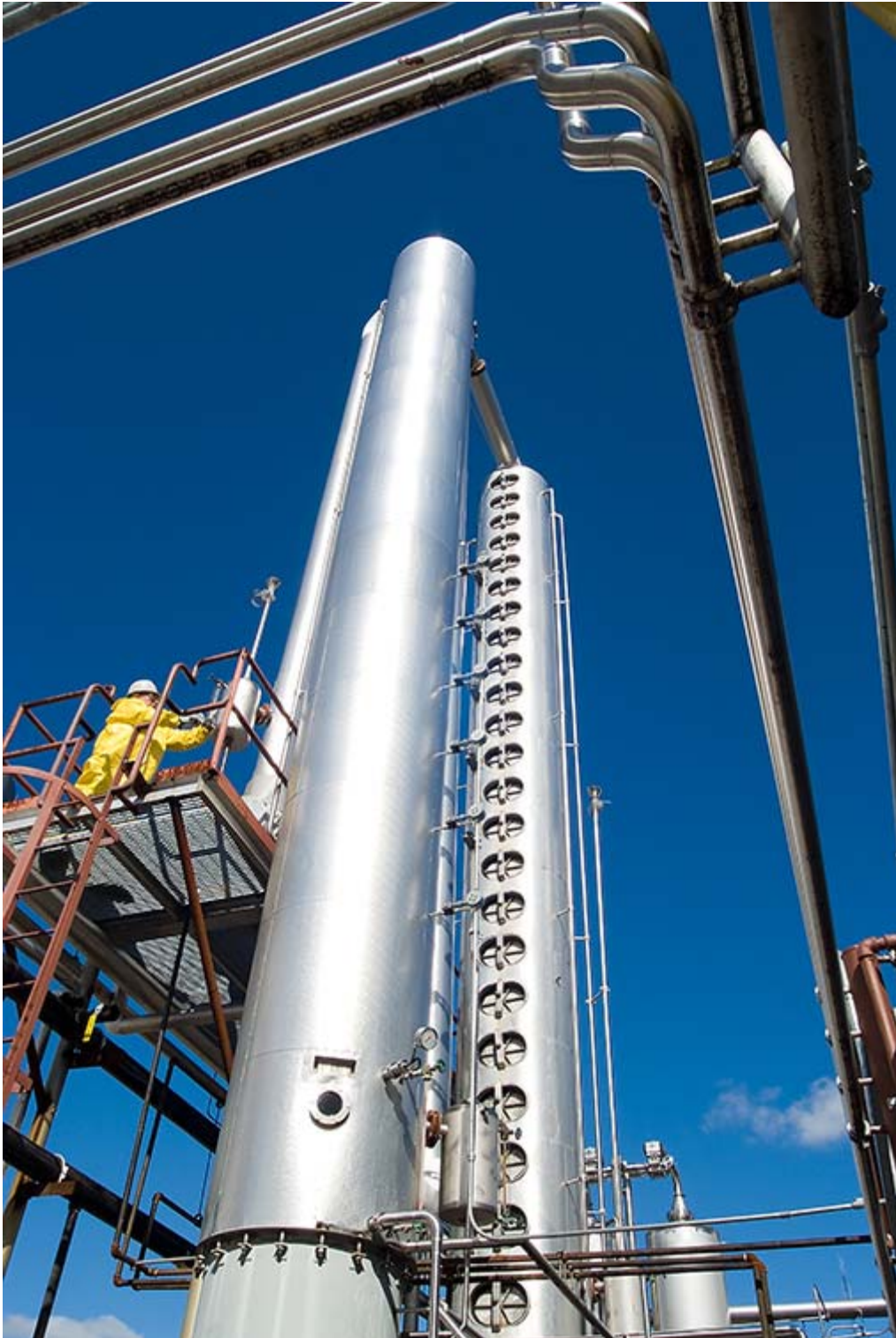
Ethanol recovery distillation unit, Veolia Environmental Services' Medina, OH
